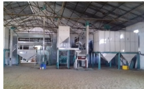
Bengal Gram Processing Facility
